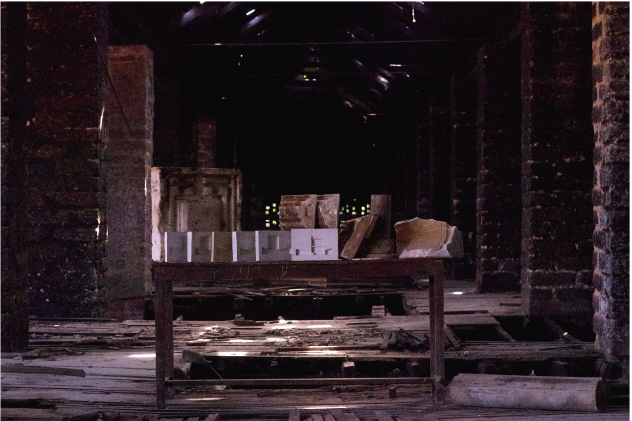
Talapady House(2019-ongoing): Wall Casts to test the design, seen in the context of a tile factory in the process of demolition Mangalore, India © A Chatterjee & A Sumra (Arijit Chatterjee and Asha Sumra. Making and Breaking: Talapady House . Mangalore, 2020: https://architexturez.net/doc/az-cf-193632 ).
