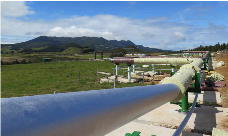
Pipeline without exterior shell showing the layer of insulation [António Franco]
